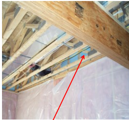
Not code compliant
