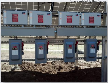
System installed by Ken Gardner
