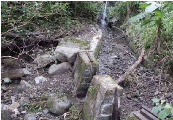
Below Settling Basin Before Cleanout - USDA Photo
