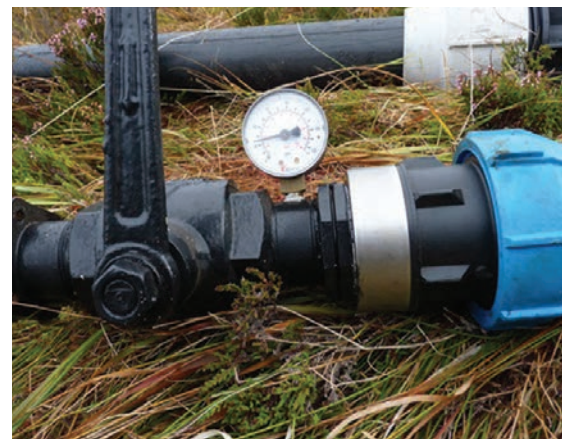
Pressure Gauge Above Turbine Stop Valve
