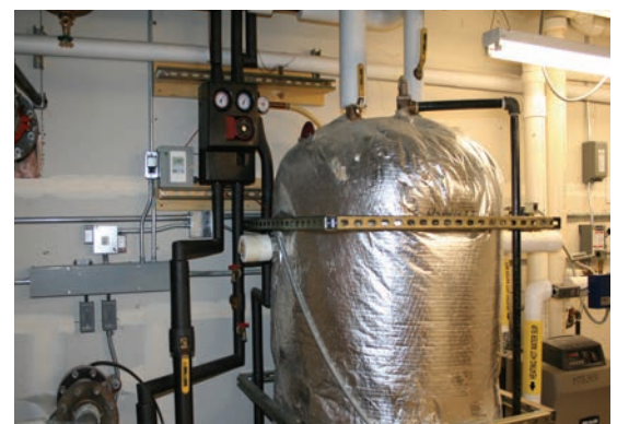
Custom Solar Hot Water Tank
