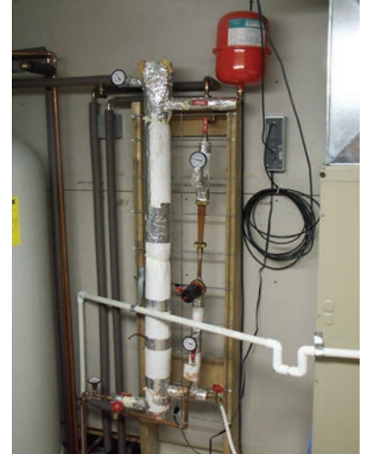
Solar Hot Water Components
