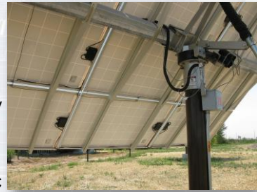
"Guarded circuit conductors?"
