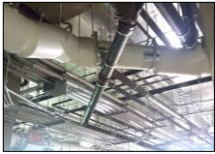
Ducts and other building systems
