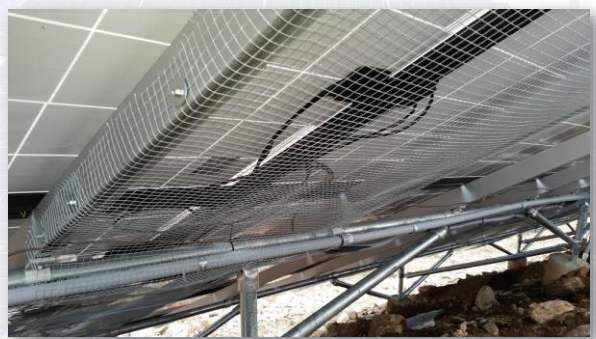
Ground-mount solar array – DC wires guarded?
