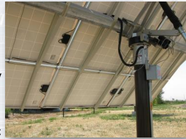
“Guarded circuit conductors?”
